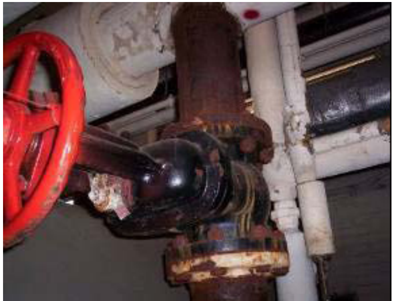
Corroded boiler and chilled water piping
