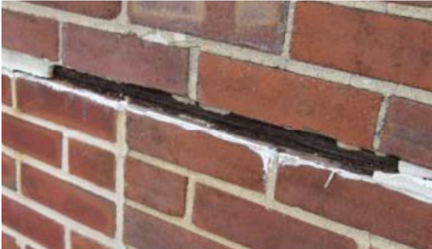
Rusting steel in upper wall causing expansion damage
