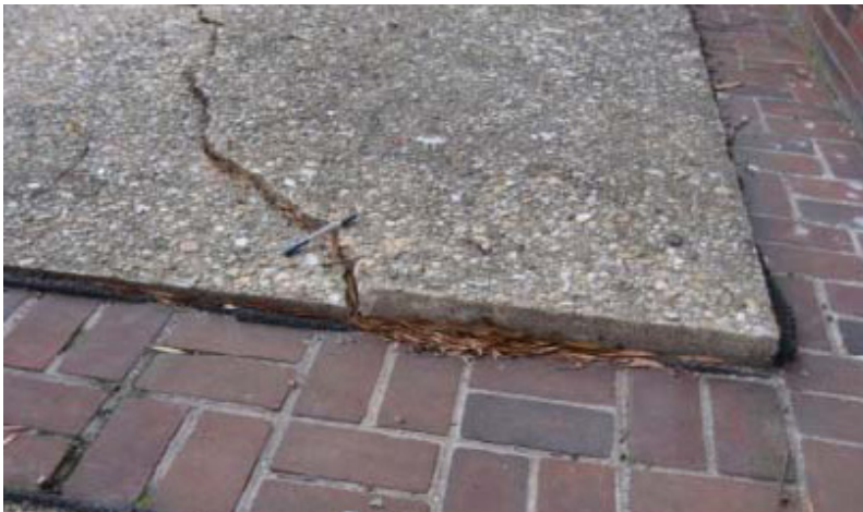
Cracked and heaved concrete in courtyard
