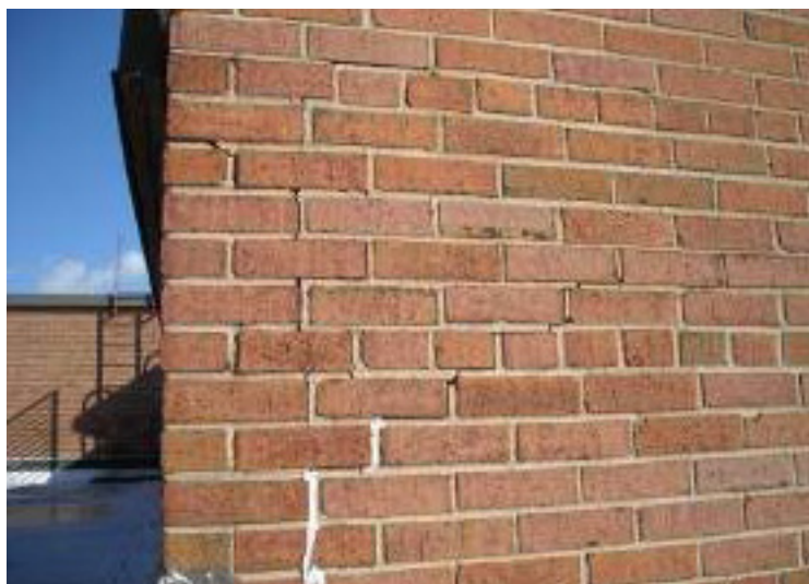
Brick masonry damaged on upper roof wall above classroom
