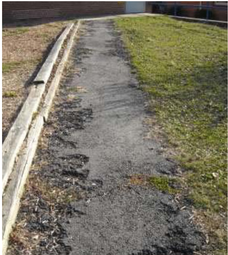
Eroded asphalt walkway
