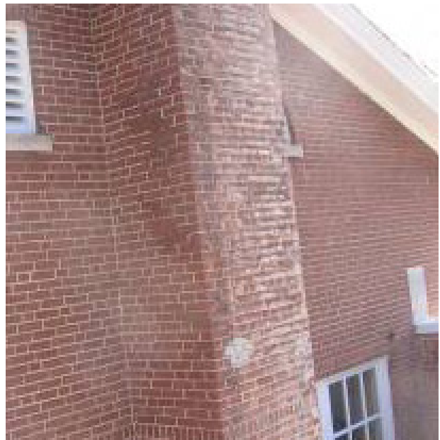
Chimney face brick masonry cracked mortar joint condition
