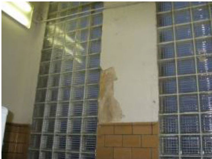
Plaster damage from chronic wall leaks
