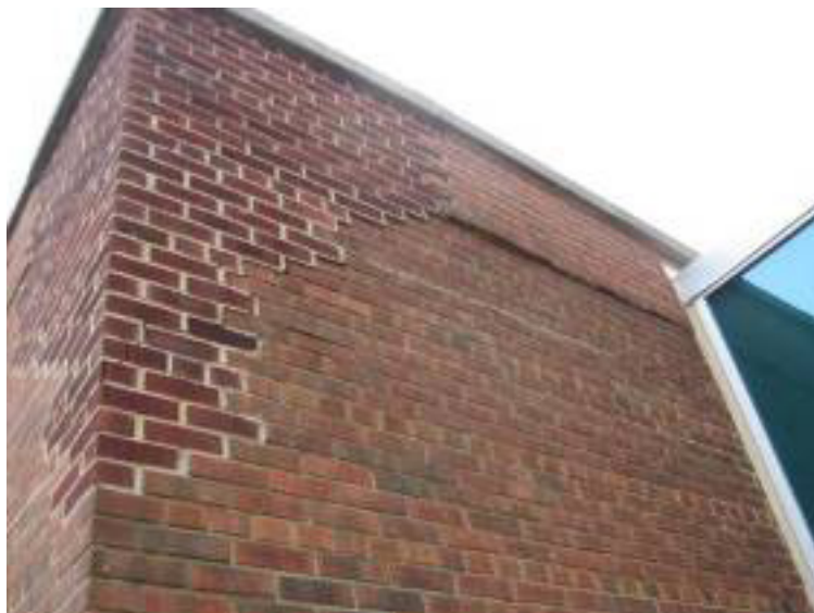
Major wall damage at gym
