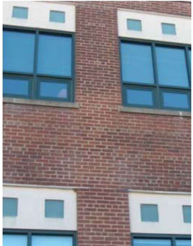
Window lintel damage and cracked mortar joints
