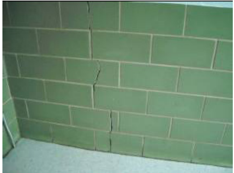
Cracked glazed terra cotta tile wall
