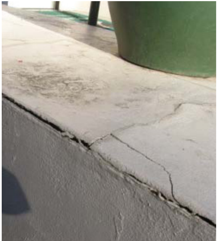
Cracks at steps
