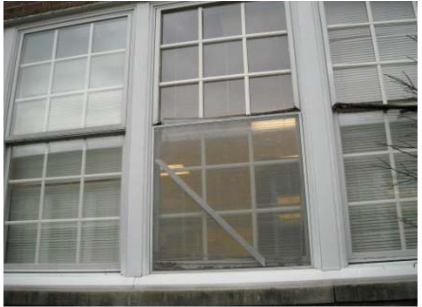
Cafeteria windows needing replacement
