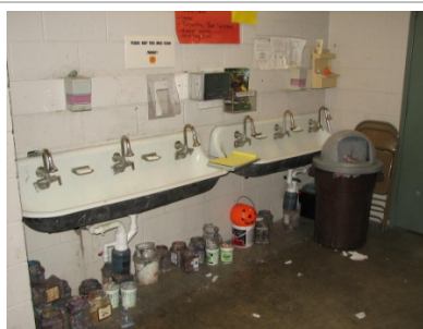
Mezzanine clean up sinks have sediment traps
